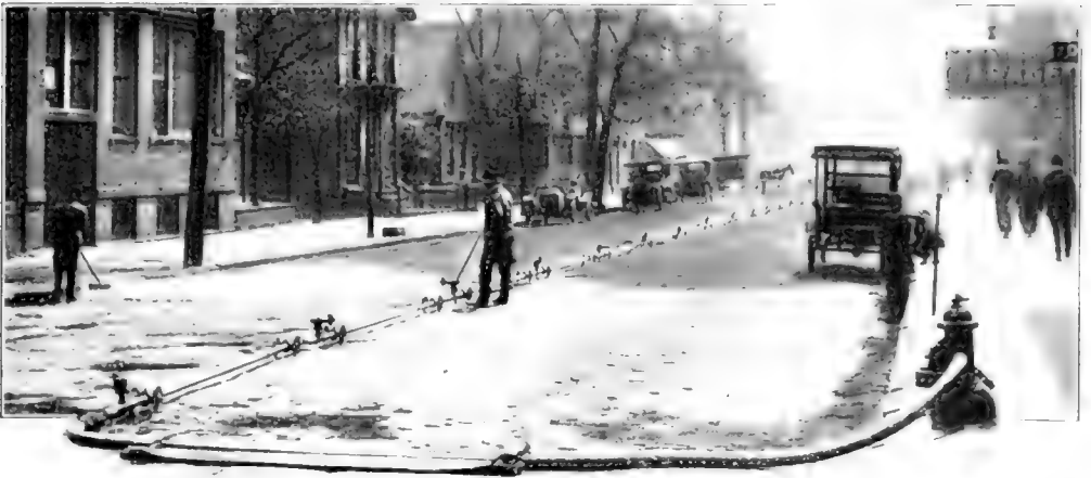
A man with a wrench opens the nozzles in succession, each stream cleaning to a line ahead of the next nozzle until the operator has gone over the entire area between hydrants
